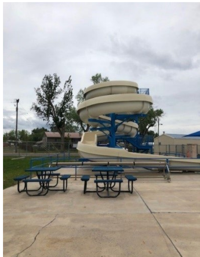
Pool slide & concrete condition
